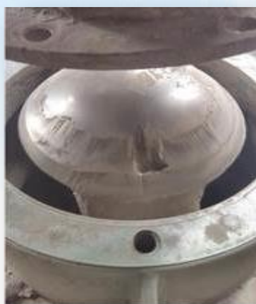
Corroded Spherical Valve
